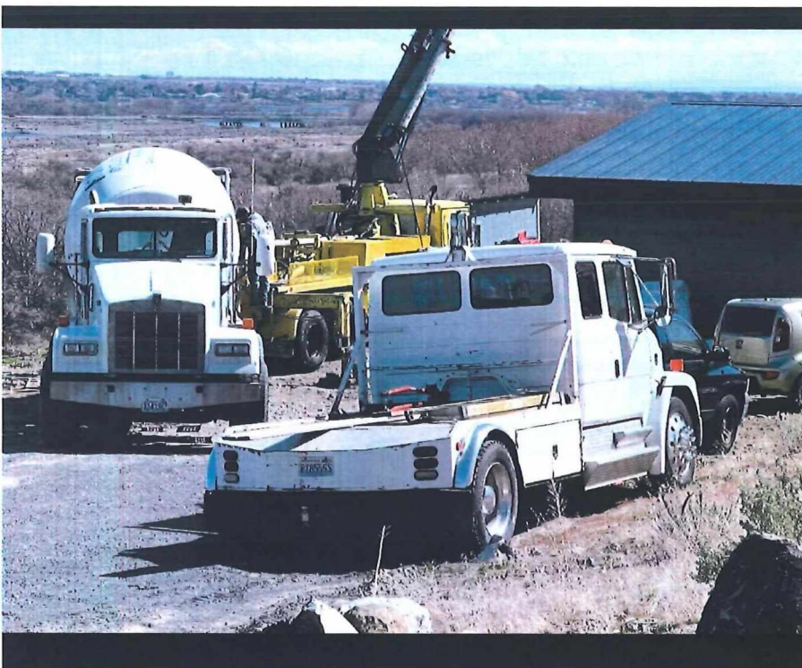
April 5, 2023 Concrete work Contractors sheared off Property stake installed January 2023
